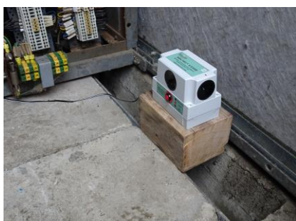
SOLTEC® V3300 in a railway signal bungalow
